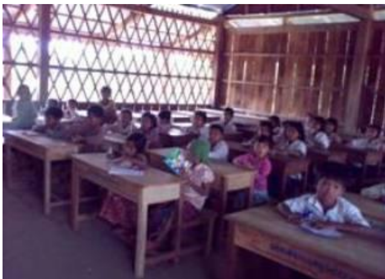
Picture 4.5 An incomplete school in Pursat province, Cambodia
